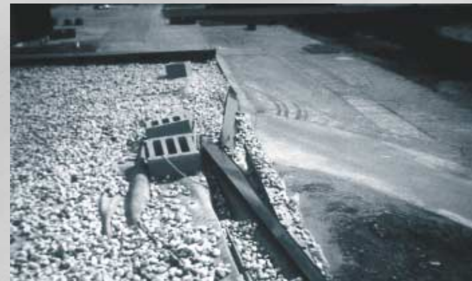
Bent and peeled flashing creates gaps for wind and water penetration
