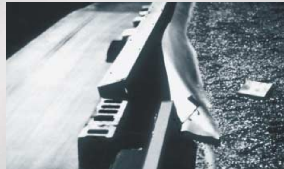
Failure of nail attachment to masonry wall.
