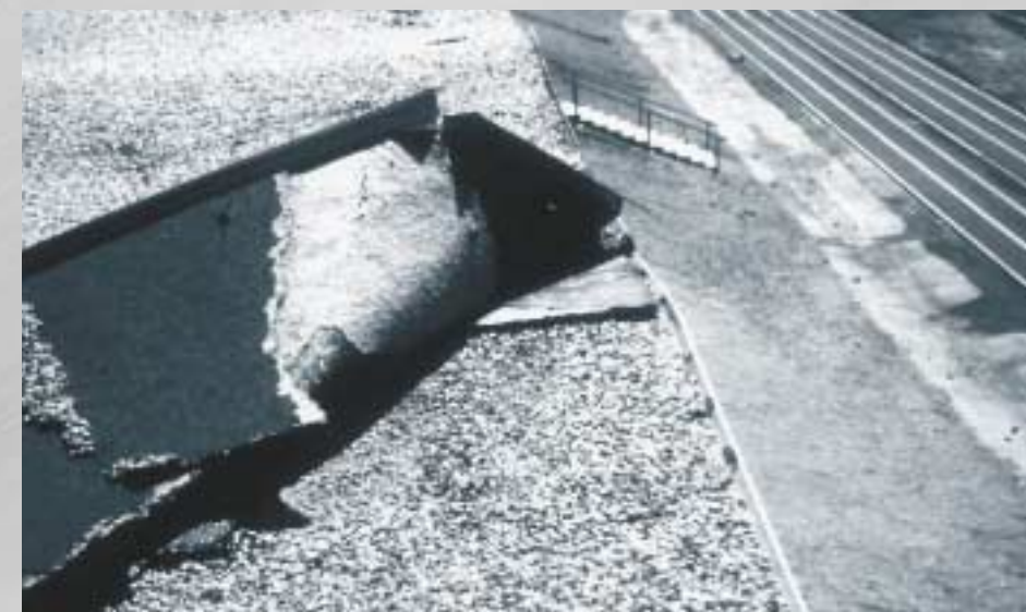
Bending and peeling of flashing takes the top layer of roof covering with it.
